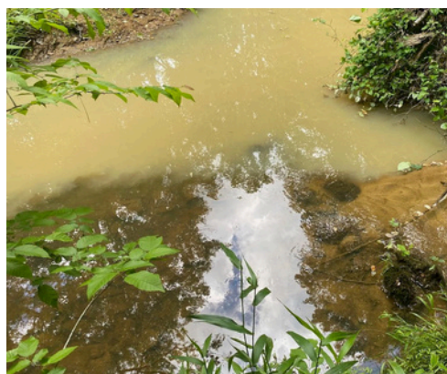
Sediment from the Moriah Energy Center construction site in Person Co. erodes into a stream. The stream flows to Lake Michie, a drinking water supply for Durham.
